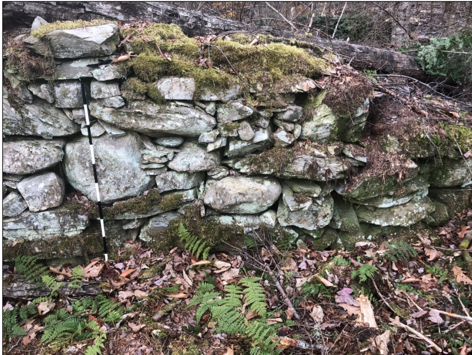
Figure 5-59. East half of intact south wall of structure at Site MP-1, facing north.
